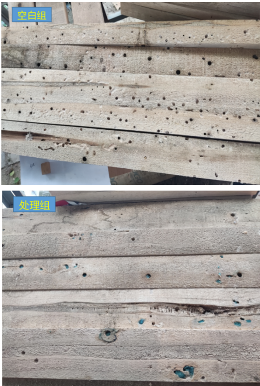
图4 北京地区固态防治药剂处理效果对比 Fig.4 Comparison of treatments of solid-state pesticide on managing carpenter bee damages in Beijing area
